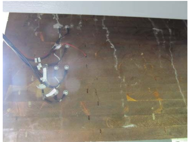
Figure 7: Measuring points of timber moisture and timber temperature at a block-glued laminated timber beam at one of the foreland bridges
