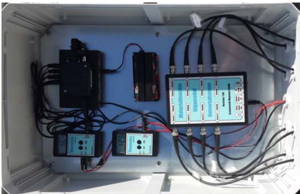
Figure 2: Measuring devices in installation box
