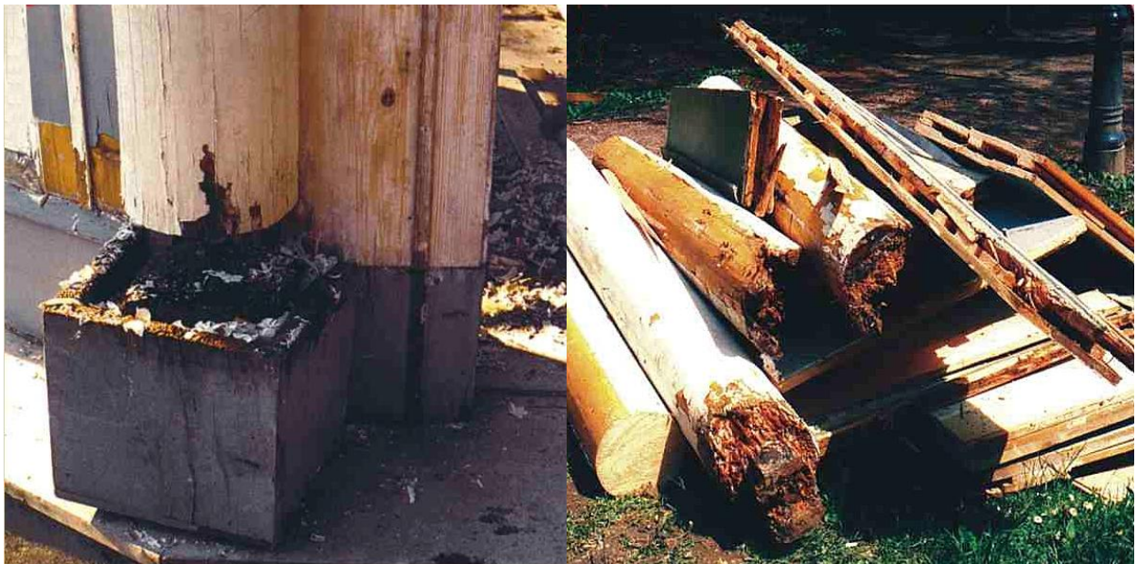
Figure 5: Decayed poles (brown rot, mainly Gleophyllum abietinum ) and soft rot found and replaced during the restoration in 2001.
