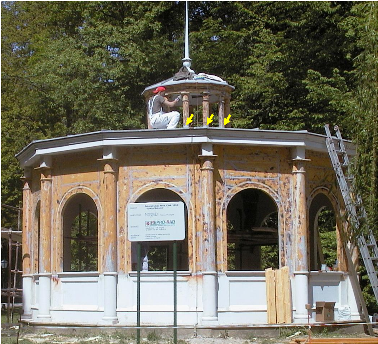
Figure 6: Restoration work in 2001. Yellow arrows: critical connection between the little top pillars and the roof sheeting.
